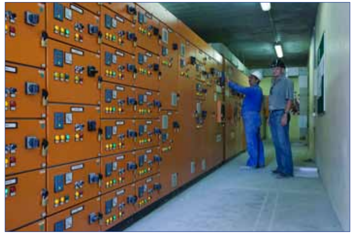
Hannes du Plessis (Electrician at Leazonia Quarry) and Gideon Roux (IRITRON) at the new MMC for the Tertiary and Roadstone Crusher Plant
